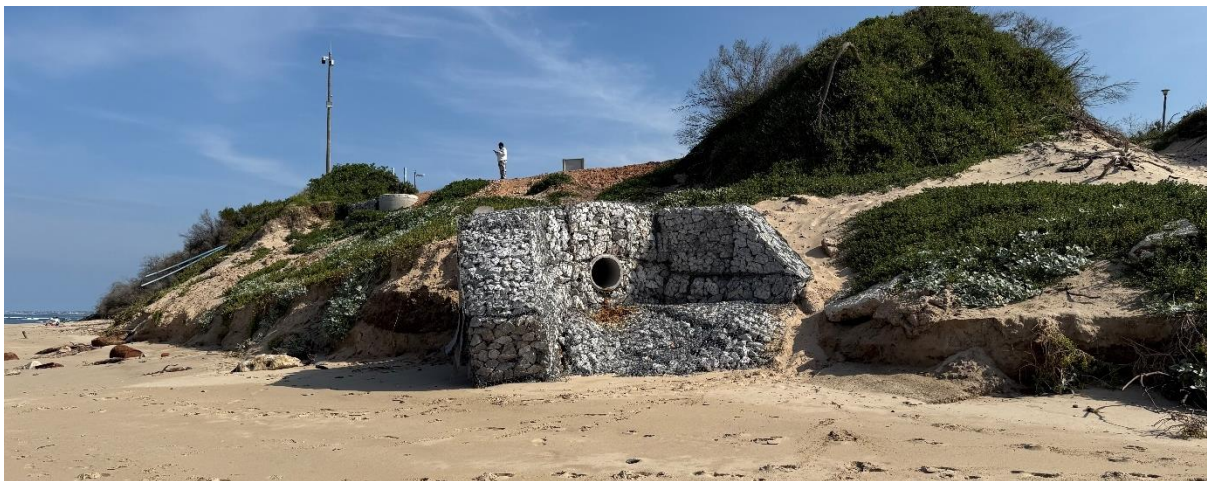
Figure 4.25: Stormwater infrastructure located along Paradise Beach
